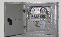
Air boiler control 3 phase
