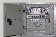
Air boiler control 3 phase
